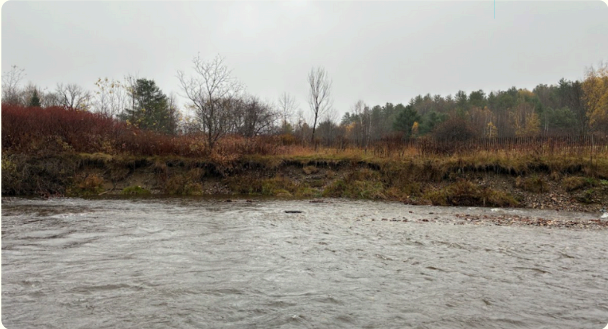
Streambank erosion at Mills Riverside Park prior to planting, facing east. (Credit: Winooski NRC D)
